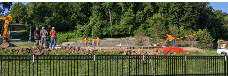
Spire employees work on the concrete pad that supports the Super Hornet display.
