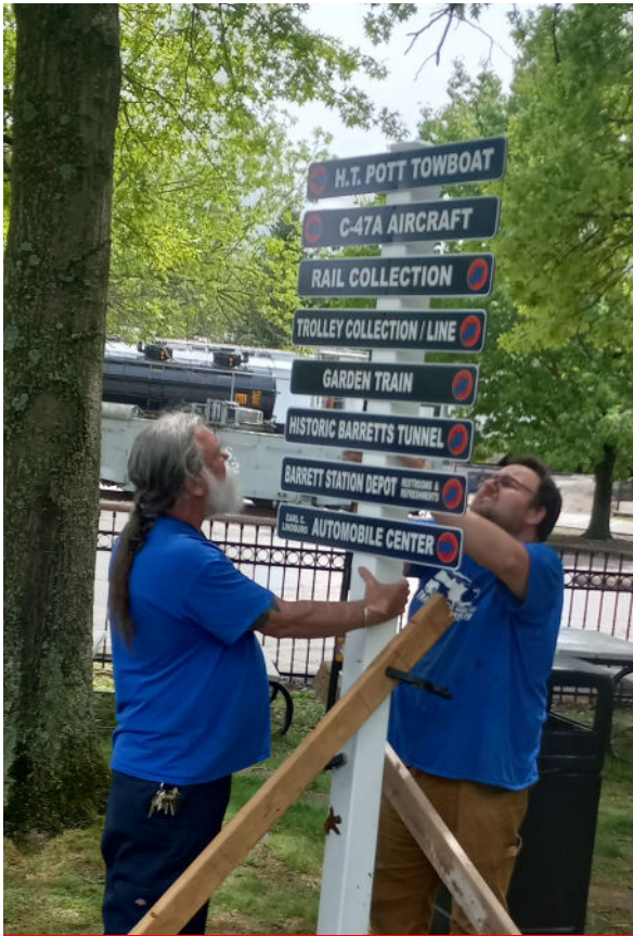
Coby Ellison and Andrew Arth install directional signage at the top of the zig-zag path.
